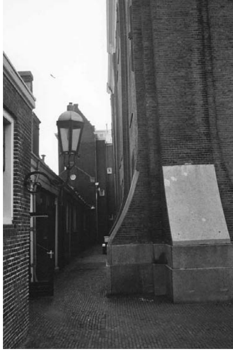
Figure 6: Section of the wall of the Portuguese synagogue, Amsterdam, in the form of the original construction in the 1670s
